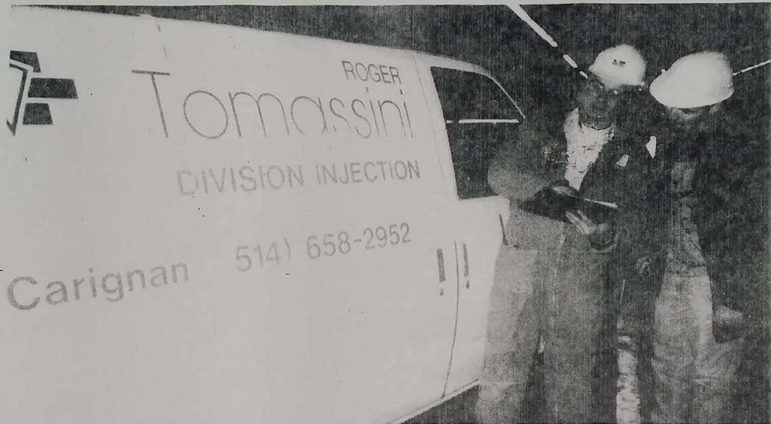
Roger Tomassini, left, goes over the game plan with one of his crew before beginning the night's work in the Lafontaine tunnel.
